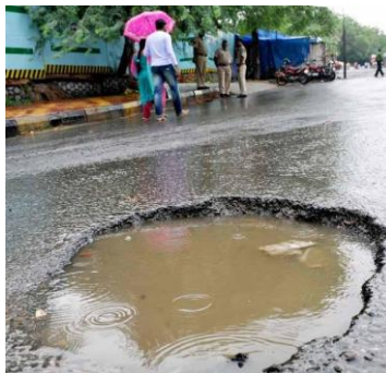
Fig. 1. Condition of roads with potholes.
